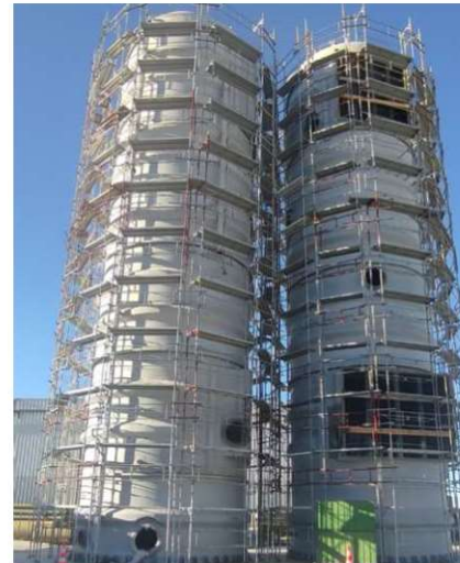
7 scrubber sectors and their piping
