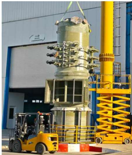
scrubber and the embedded piping.
