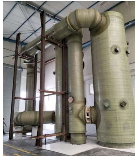
Scrubbers and ducts
