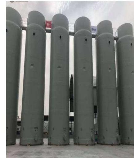
Cascade of tanks with adjacent platforms
